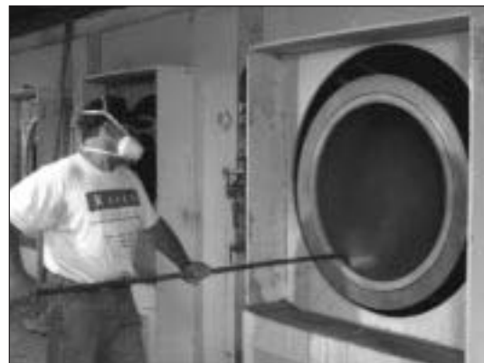
Each layer of glass and resin is rolled to remove air bubbles and to insure a dense uniform laminate.
