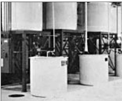
Industrial waste water treatment facility.
