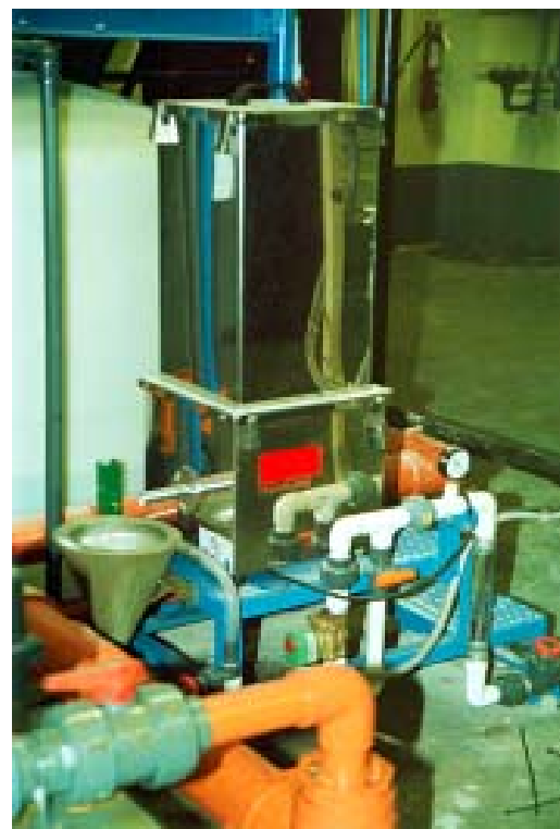
DRY POLYMER MIXING SYSTEM
